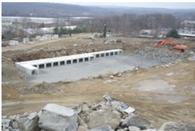
Figure 1. Underground storm water retention basin under construction in January 2010. The walls exposed mostly amphibolite bedrock, but glacial till was exposed in the corner at far left (Harold Moritz photo).
